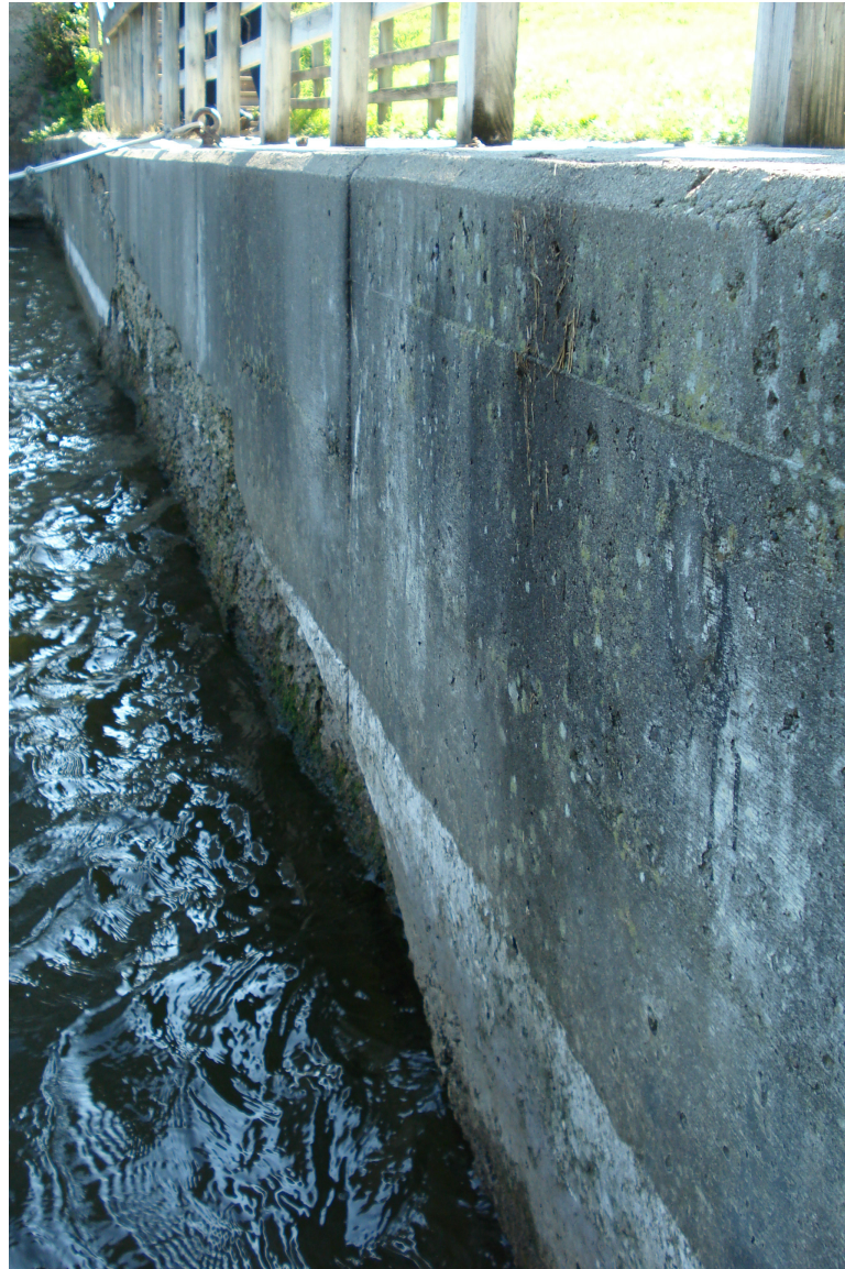
Downstream Left Wing Wall – Cores shall be taken into the vertical face of the downstream left wing wall just above the water line.
