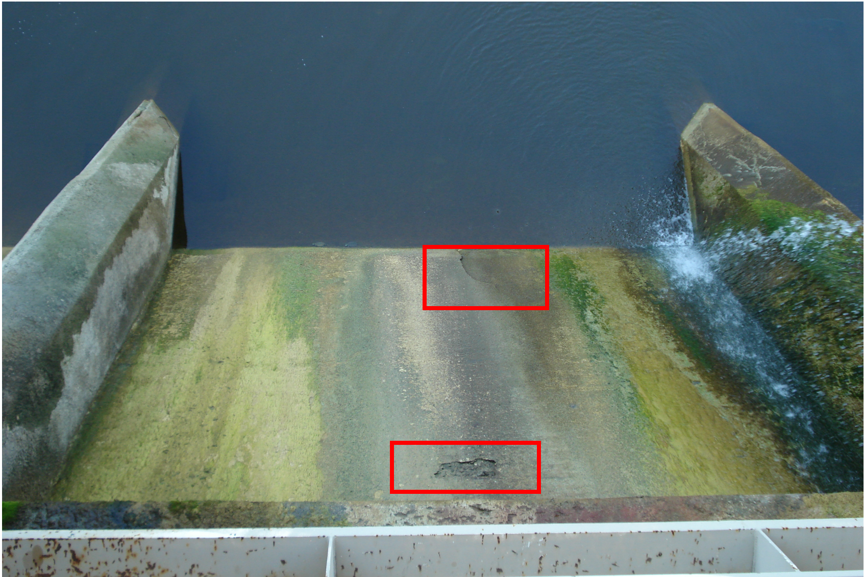
Spillway Face – Cores shall be taken into the spillway face. Shown above is the spillway face looking down from the walkway on top of the dam.
