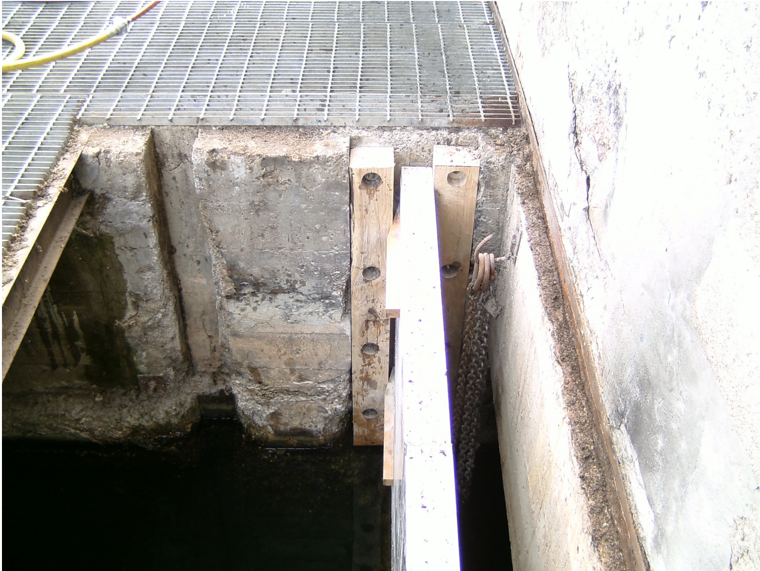
Intake Structure – View with grating removed. Cores shall be taken into the vertical faces of the intake structure beneath the grating.
