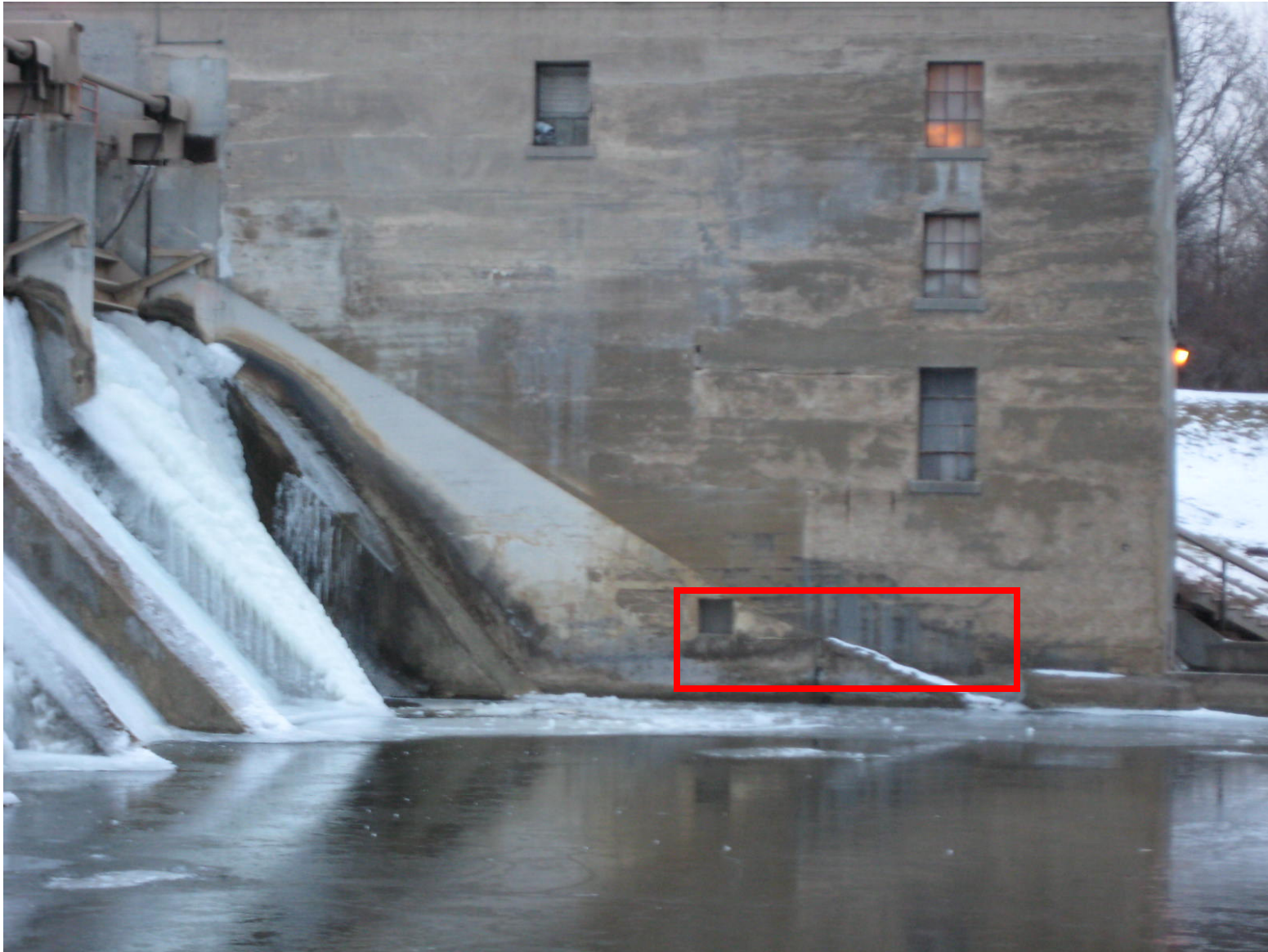
Power House – West wall. Cores shall be taken into the vertical face of the Power House West Wall.
