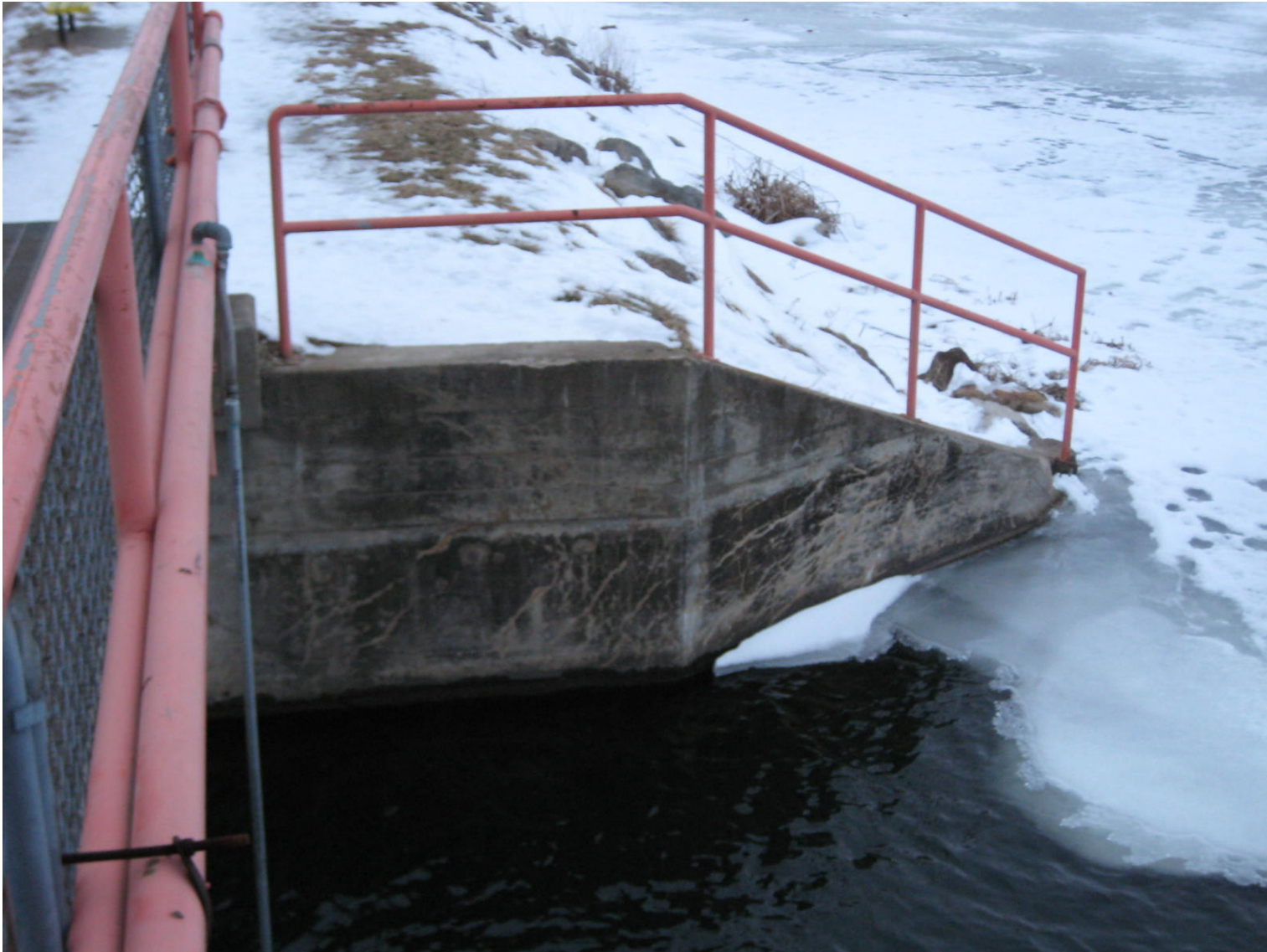
Upstream Right Retaining Wall – Cores shall be taken into the vertical face of the upstream right retaining wall just above the water line.
