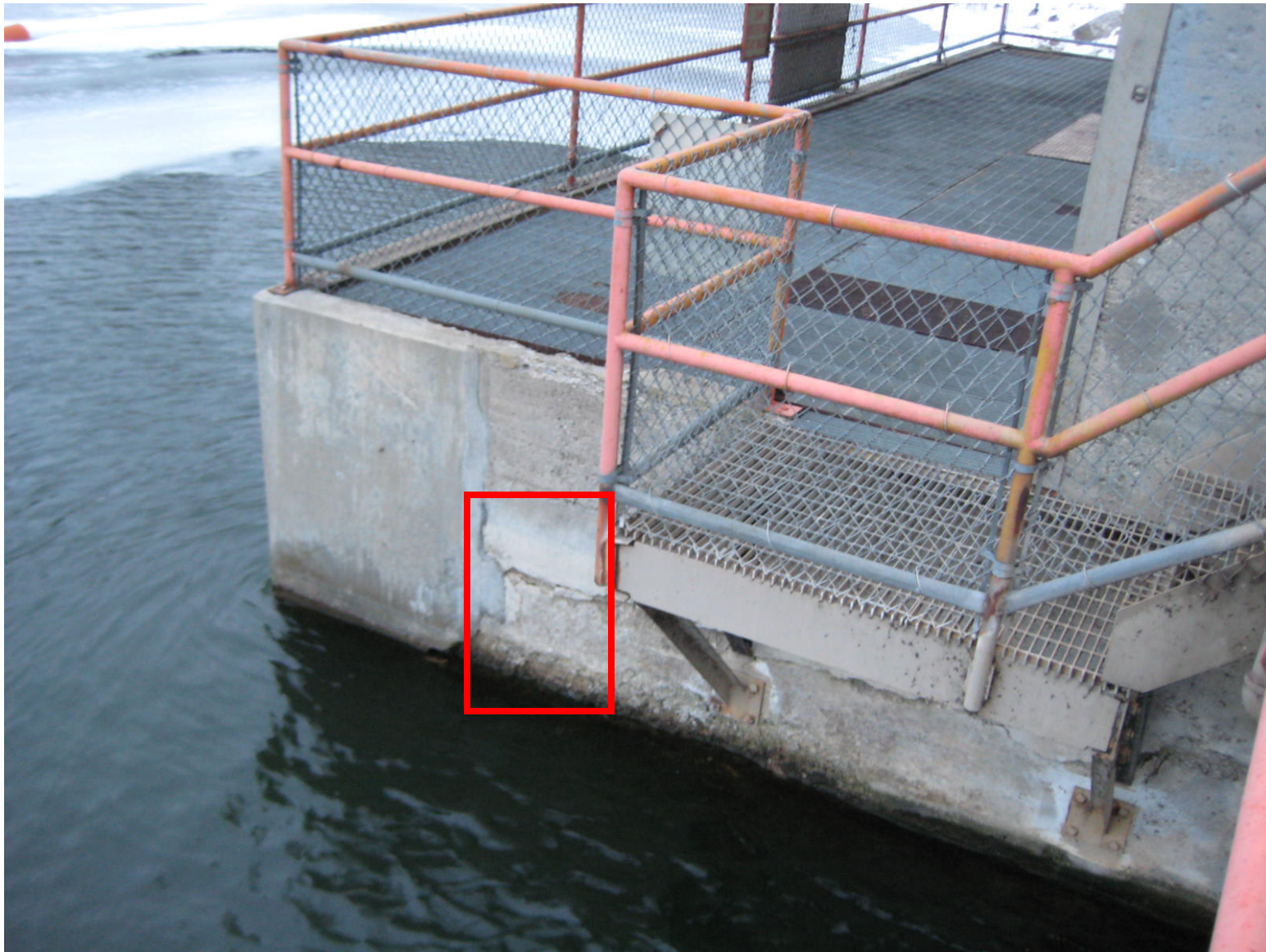
Intake Structure – West wall. Core shall be taken into the vertical face of the intake structure just above the waterline.
