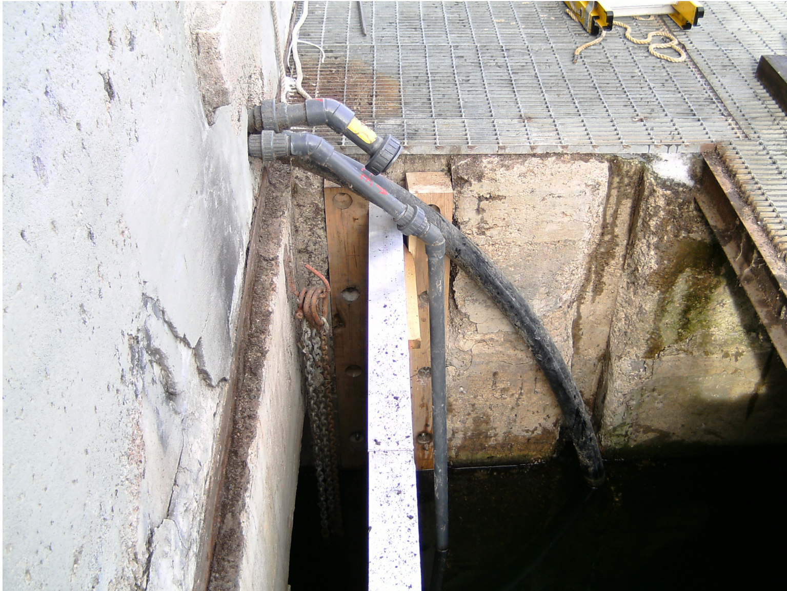
Intake Structure – View with grating removed. Cores shall be taken into the vertical faces of the intake structure beneath the grating.
