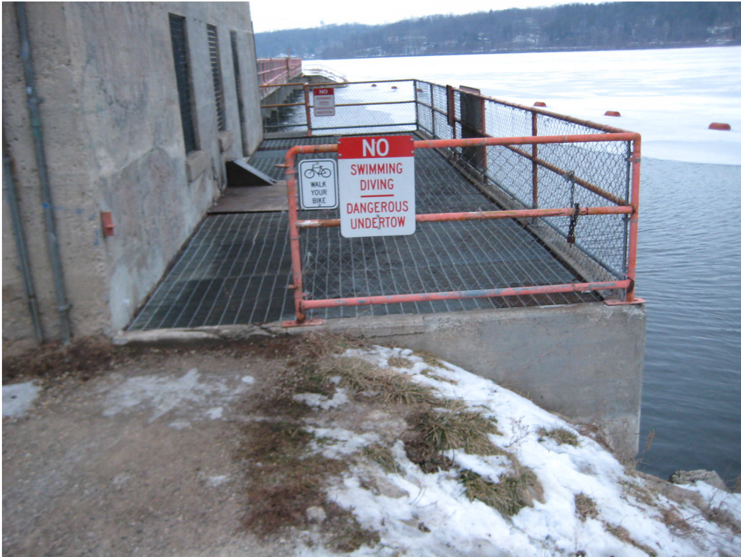
Intake Structure – View from the east. Cores shall be taken into the vertical faces of the intake structure beneath the grating. Removal and replacement of the grating will be required.
