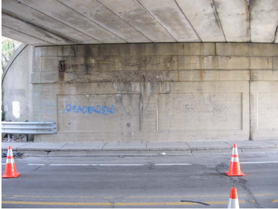
Photo 5: Picture showing north half of east abutment with delaminated areas and cracks.
