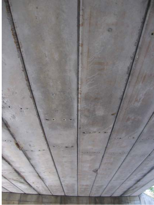
Photo 13: Picture showing west side of bottom of beams with spalled concrete and exposed reinforcing strands on north side of bridge.
