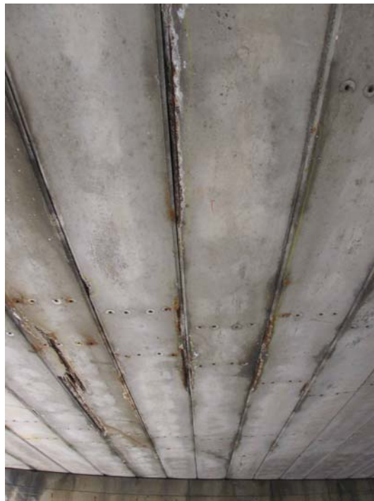
Photo 12: Picture showing west side of bottom of beams with spalled concrete and exposed reinforcing strands at center of bridge.
