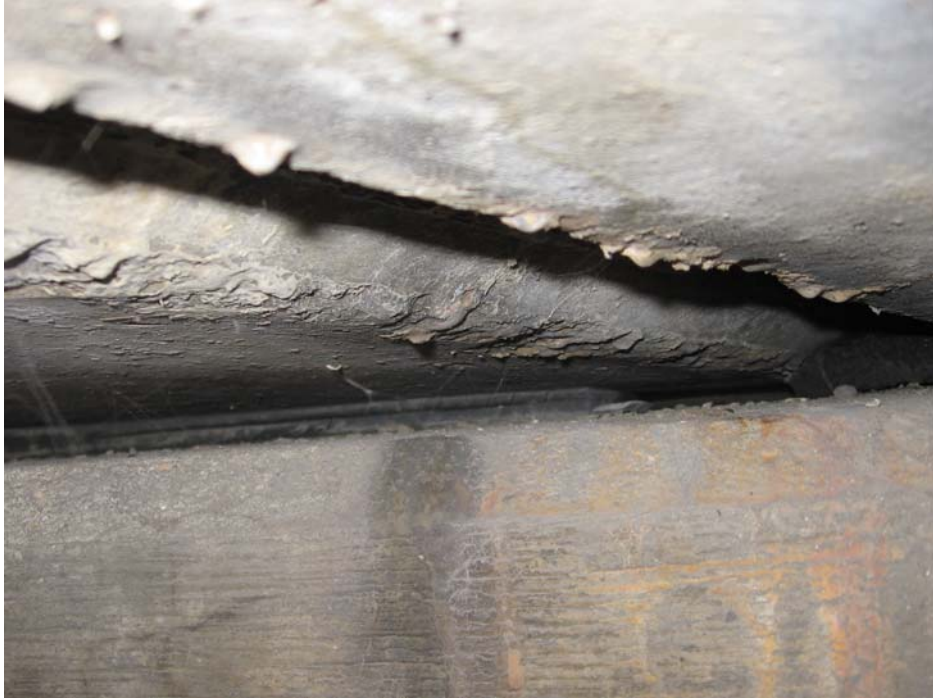
Photo 15: Picture showing bearing pad on east abutment in good condition.
