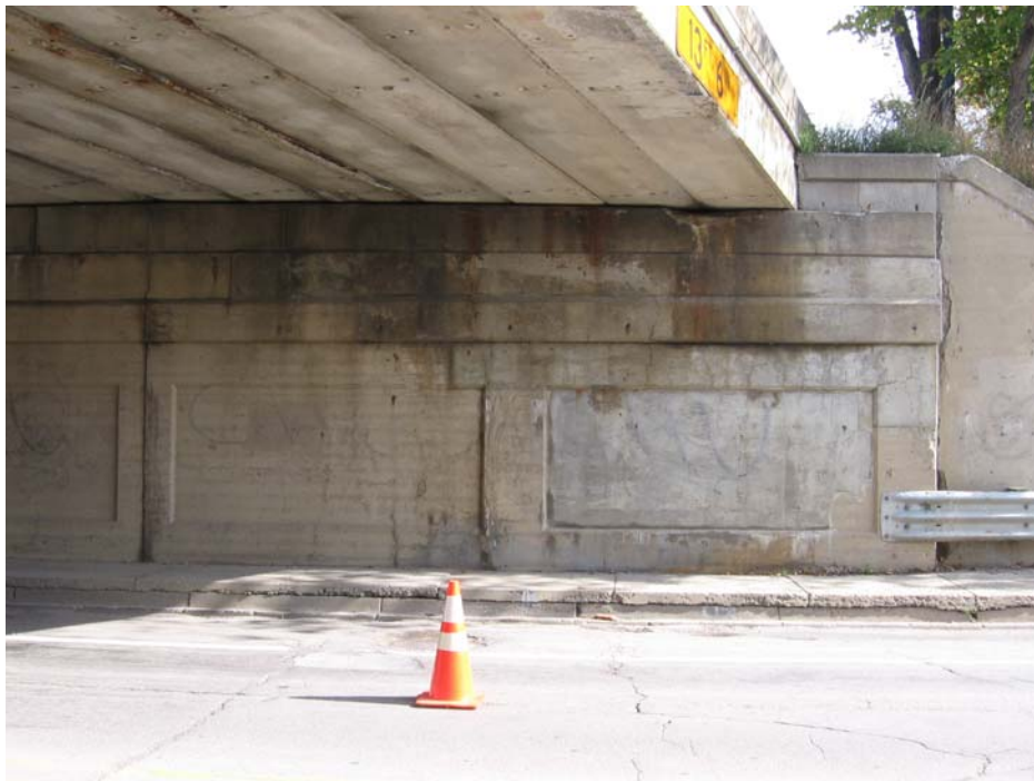
Photo 6: Picture showing south half of east abutment with delaminated areas and cracks.
