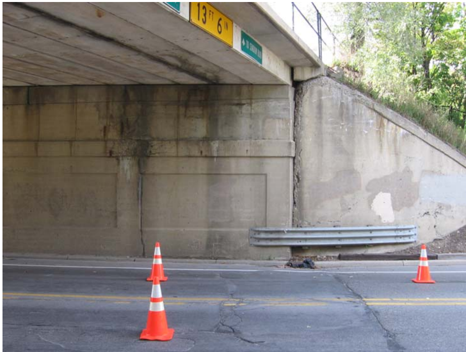
Photo 7: Picture showing north half of west abutment with delaminated areas and cracks.
