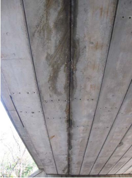
Photo 9: Picture showing east side of bottom of beams with spalled concrete and exposed reinforcing strands on north side of bridge.
