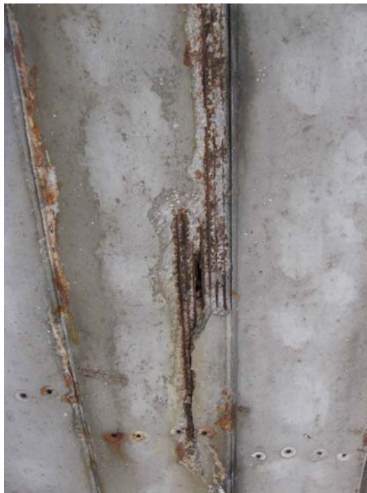
Photo 14: Picture showing bottom of beam with spalled concrete, multiple reinforcing strands exposed, and a hole to the center of the box.
