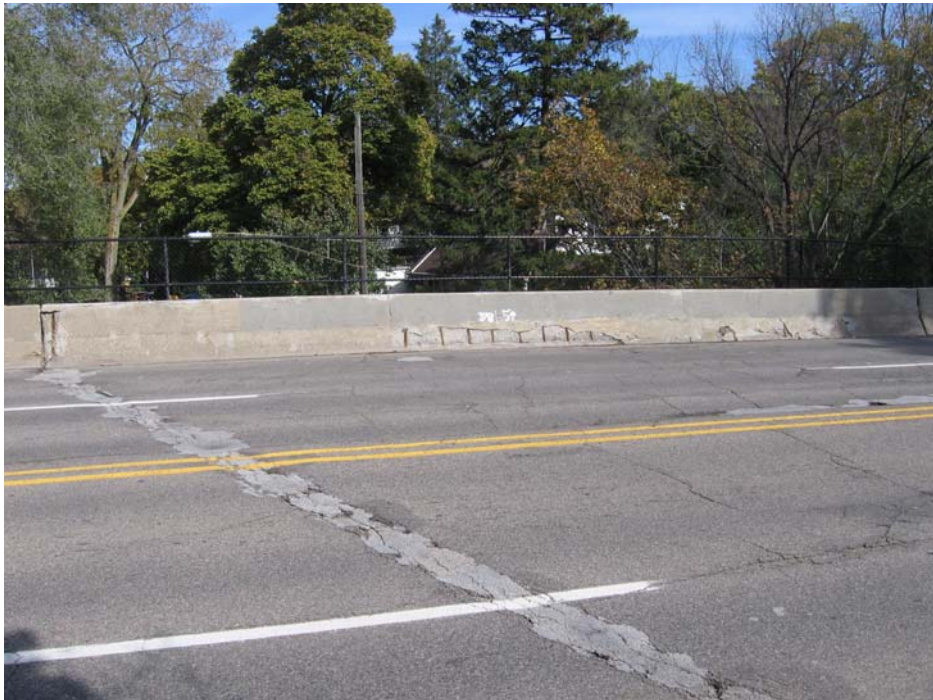
Photo 16: Picture showing spalled concrete and exposed rebar on north barrier.
