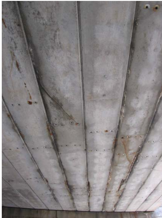
Photo 10: Picture showing east side of bottom of beams with spalled concrete and exposed reinforcing strands on south side of bridge.
