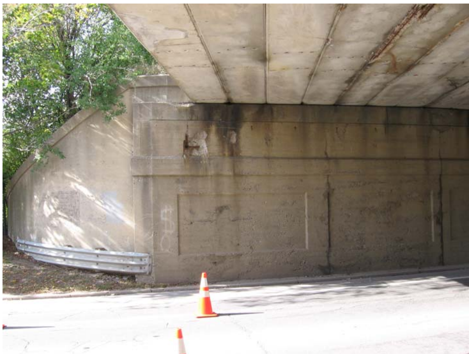
Photo 8: Picture showing south half of west abutment with spalled concrete, exposed rebar, delaminated areas, and cracks.
